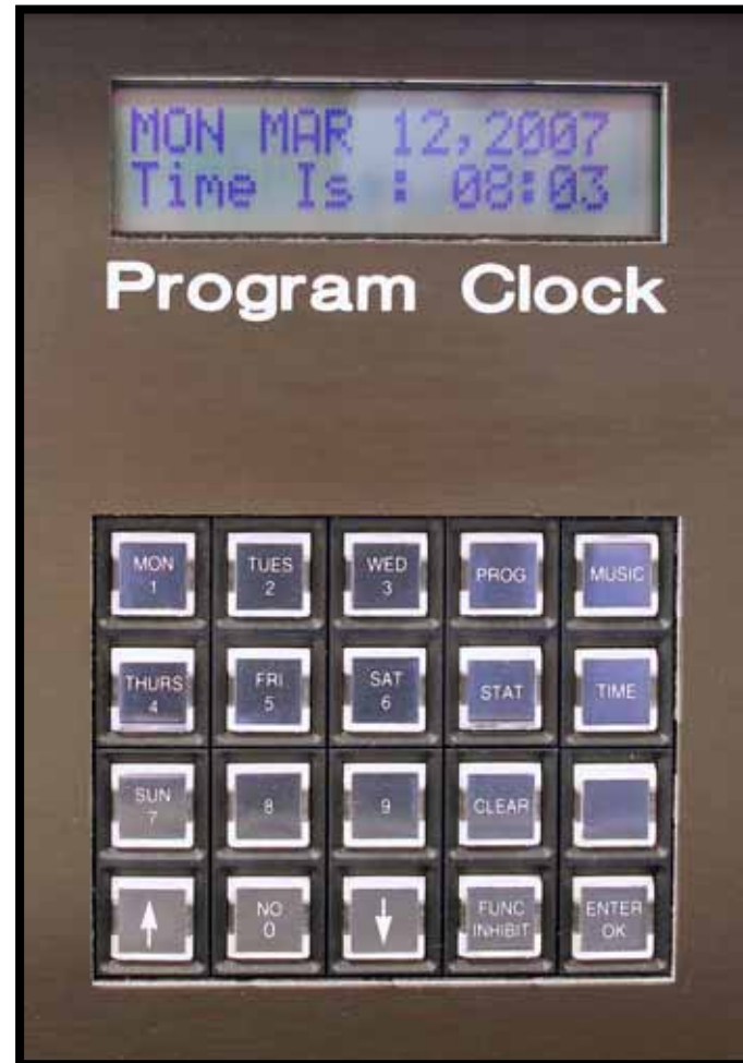
Close up view of controls
